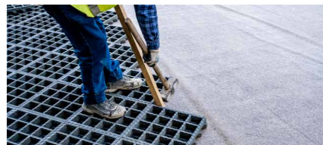
Ensure tight installation and regular tapping to prevent later forming of gaps.
